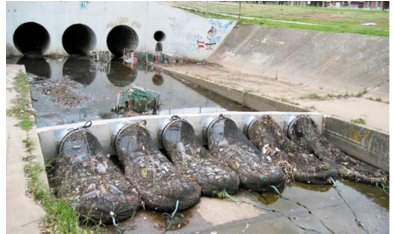
Image 6.3- Stormx capture systems
