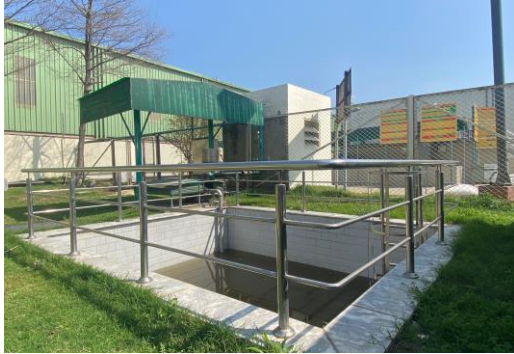
Treated Process Wastewater Storage Tank for Reuse
